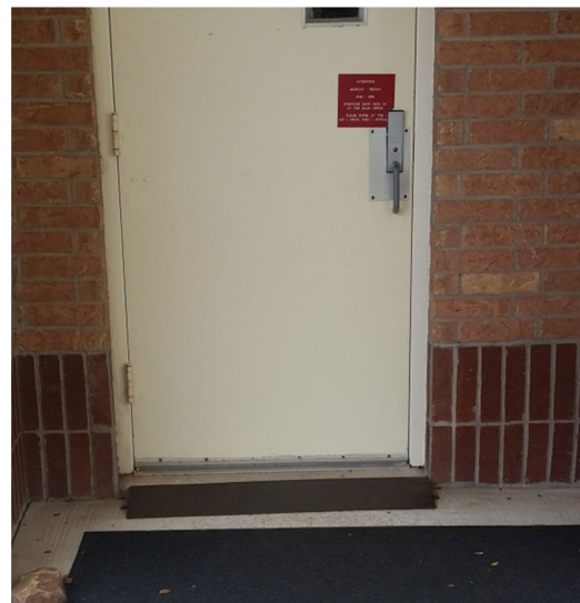
Figure 8: un-accessible threshold at west entry door.
