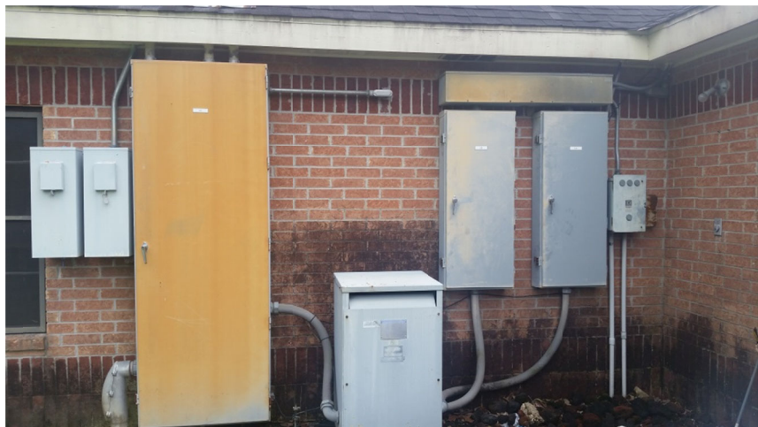
Figure 10: MDP, transformer, and service panels.
