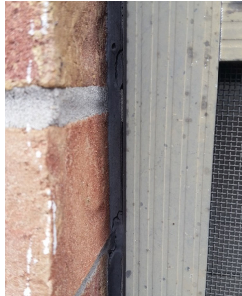
Figure 2: Caulk splitting and separating from window.
