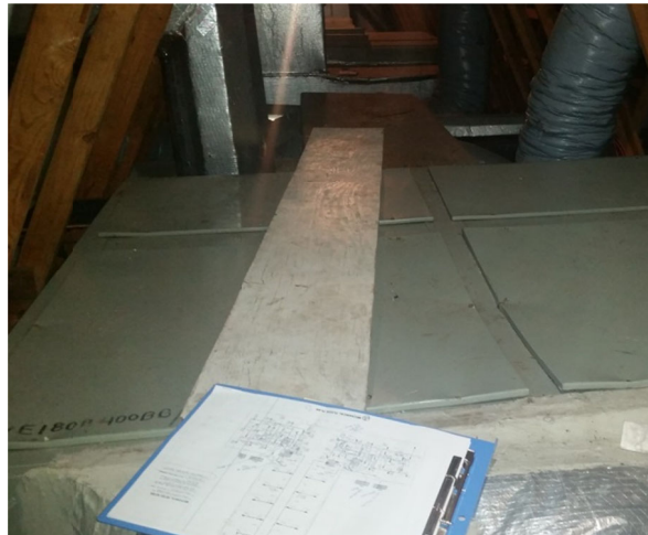
Figure 9: a board is used to walk across top of AHU in attic.
