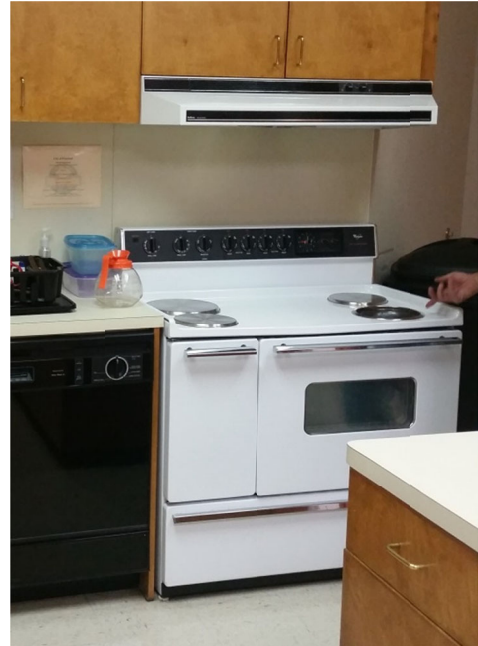
Figure 6: range with heating elements removed.
