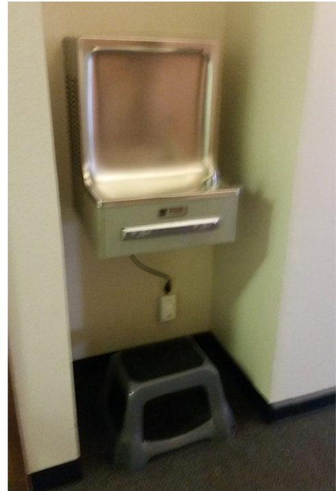
Figure 7: drinking fountain is not accessible.
