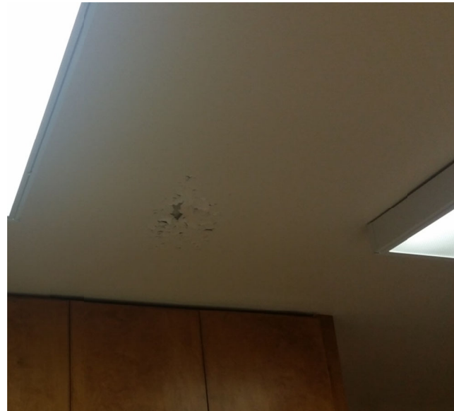
Figure 5: Peeling paint on Kitchen ceiling
