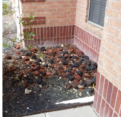
Figure 4: mulch and landscape rocks applied directly against weep openings.
