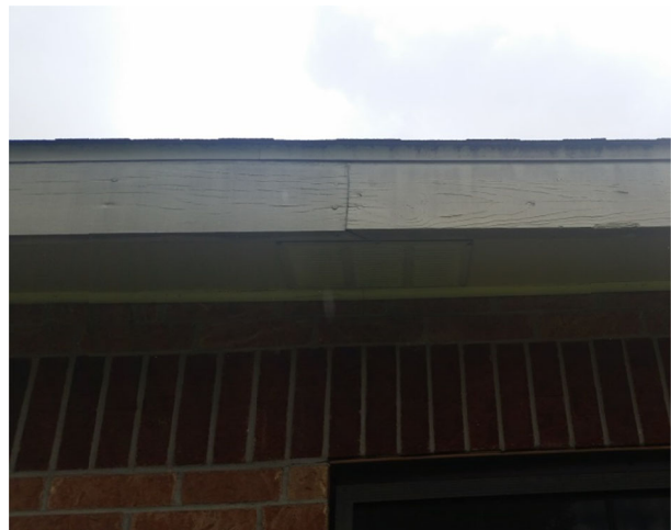
Figure 1: Water damage seen on existing fascia; weep joints missing at lintel.
