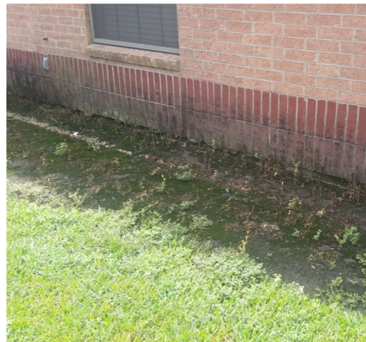
Figure 3: Poor drainage near foundation.
